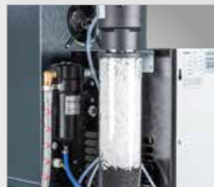
· Condensate conditioner for oil-water separation
