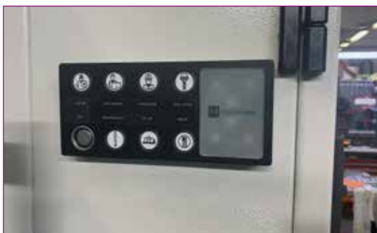
Maintenance system for monitoring machine utilisation
